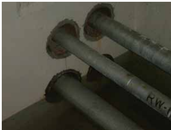
Location where the pipes penetrate through the wall between the reactor coolant filtering system spent resin storage tank room and the spent sludge storage tank room (under the water)
