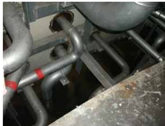
Location where the pipes penetrate through the wall between the radiation waste underground storage facility building and the radiation waste treatment building (under the water)
