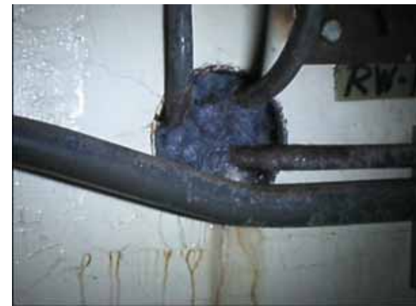
Water exuded on the location where the pipe penetrates through the south wall of the spent sludge tank A
