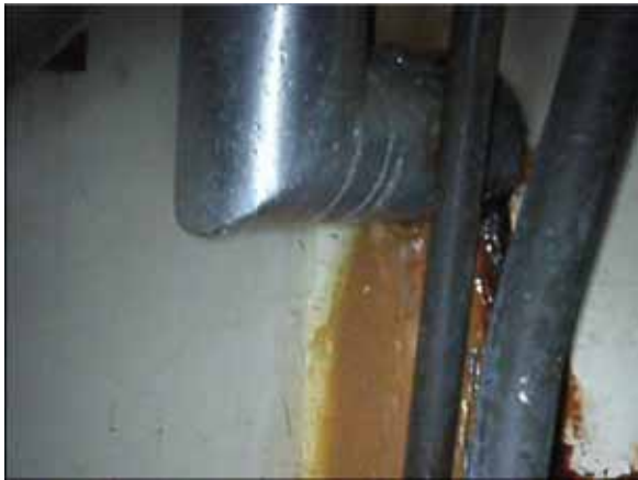
Location where water flow was confirmed on the Centralized Environment Facility Radiation Waste Common Duct (Water amount: Width of 3 fingers, No change)
