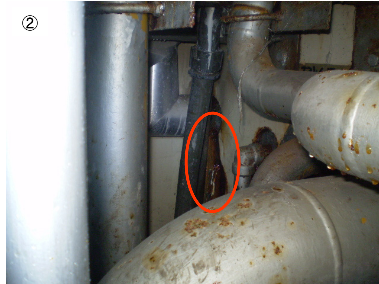
The location where the water inflow was confirmed
