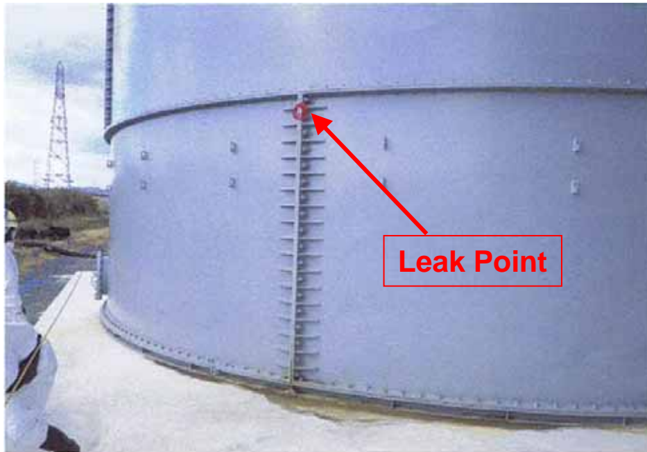
< Tank that occurred leakage >
