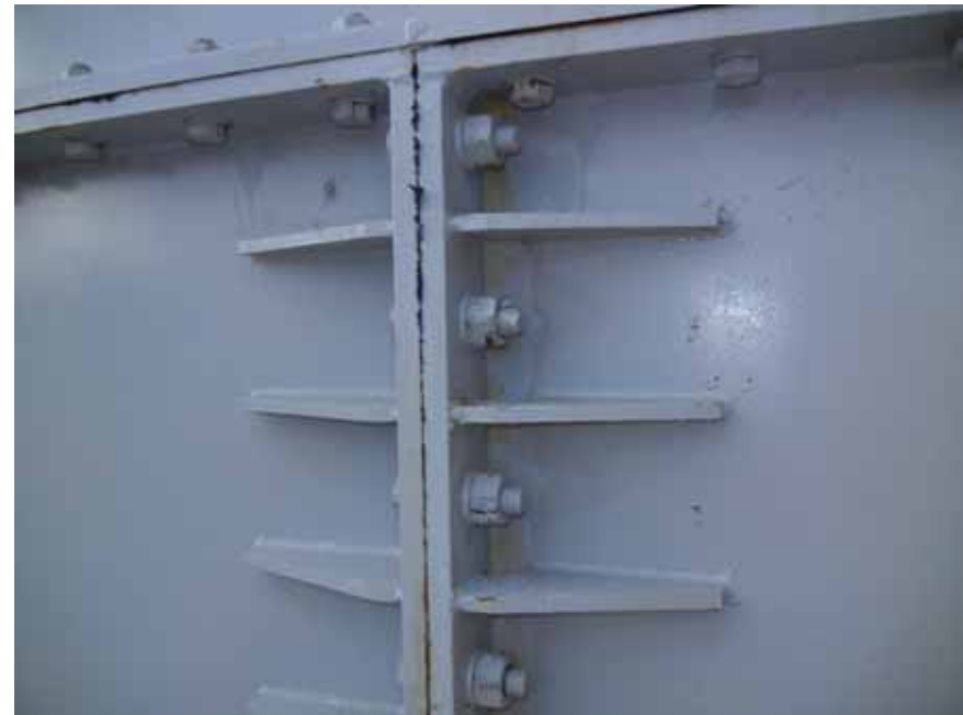
< After additional clenching, it stopped to leak >
