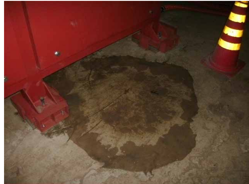
The situation of water leakage
