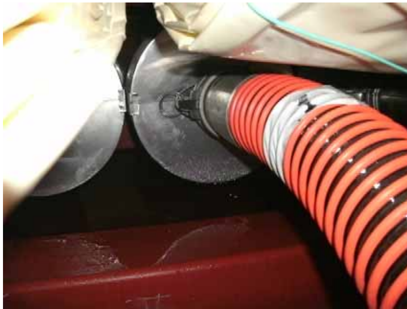
The situation of water leakage
