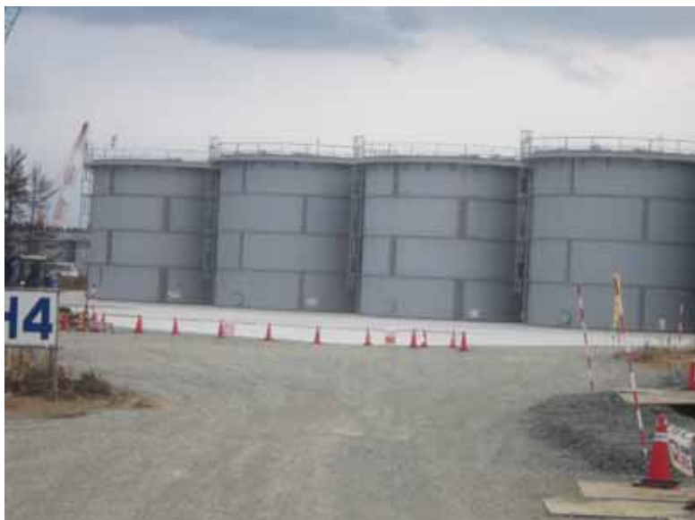
- 1 Tank array at H area Jan. 9, 2012 photo by TEPCO staff
