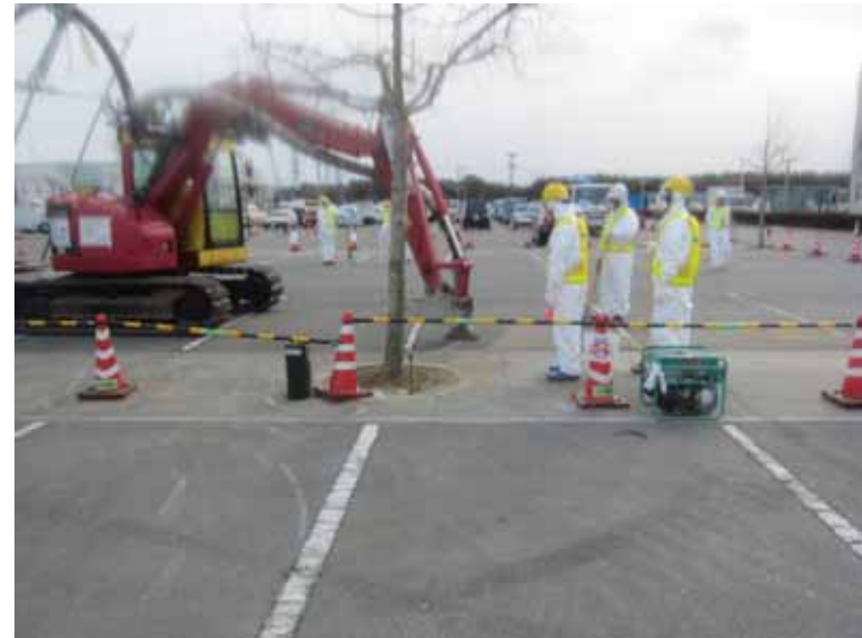
- 5 Collection work of dust and small debris at parking area of Main Anti-earthquake Building Jan. 9, 2011 photo by TEPCO staff
