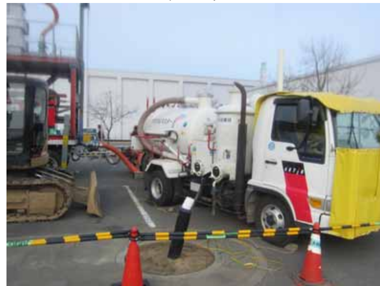
- 3 Collection work of dust and small debris at parking area of Main Anti-earthquake Building
