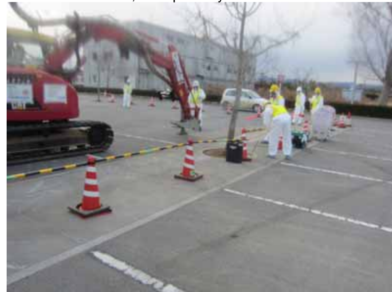
- 6 Collection work of dust and small debris at parking area of Main Anti-earthquake Building Jan. 9, 2011 photo by TEPCO staff
