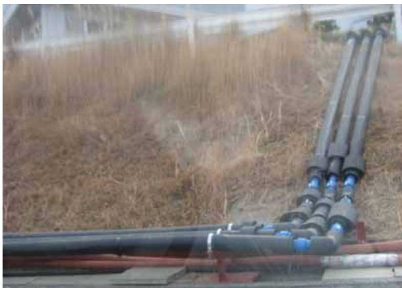
Anti-freezing measure for the reactor injection hose Jan. 9, 2012 photo by TEPCO staff
