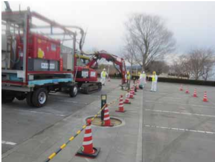
- 7 Collection work of dust and small debris at parking area of Main Anti-earthquake Building
