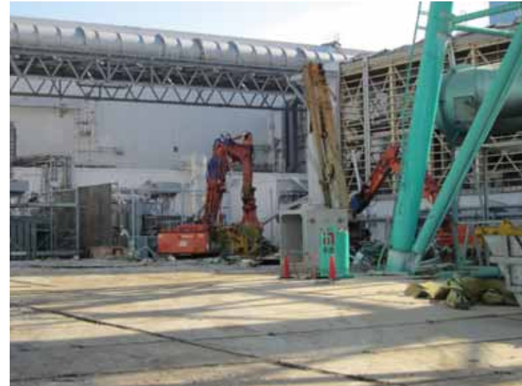
- 2 Removal of debris around Unit 3,4 Reactor Building Jan.10, 2012 photo by TEPCO staff
