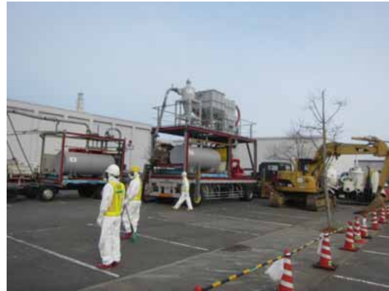
- 2 Collection work of dust and small debris at parking area of Main Anti-earthquake Building
