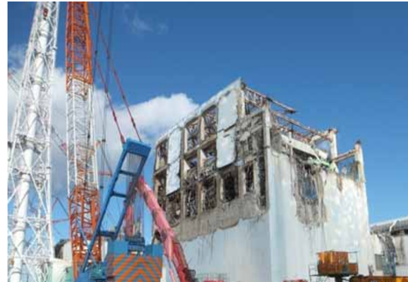
- 8 Removal of debris on the upper side of Unit 4 Reactor Building (after work)
