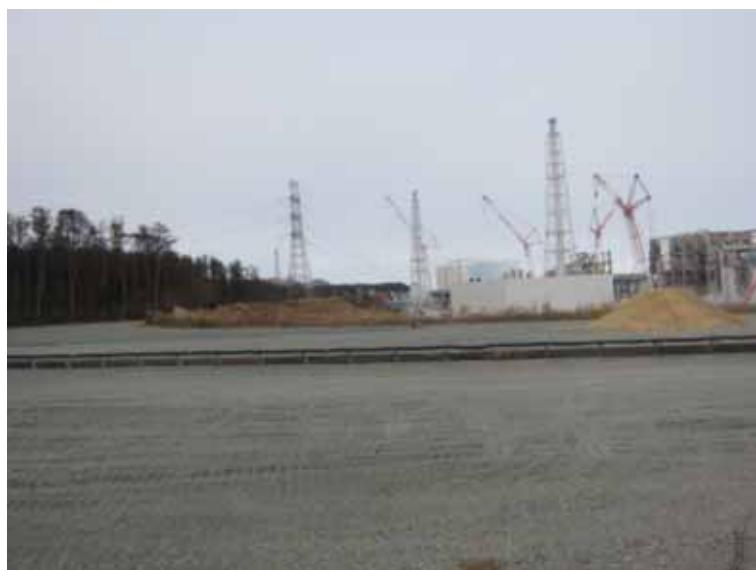
- 3 Look into Reactor Building from the hill in the southern side of Unit 4 Jan. 9, 2012 photo by TEPCO staff
