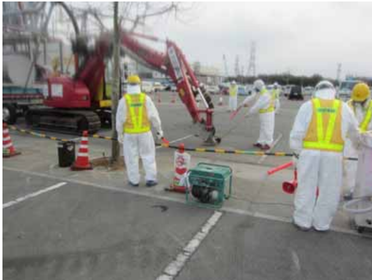
- 4 Collection work of dust and small debris at parking area of Main Anti-earthquake Building Jan. 9, 2011 photo by TEPCO staff
