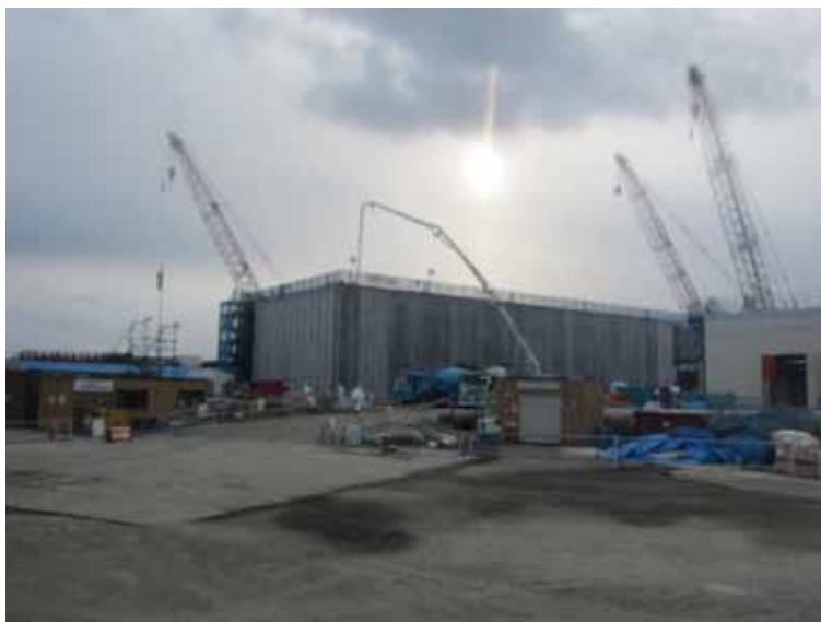
- 2 Waste sludge storage facility Jan. 9, 2012 photo by TEPCO staff
