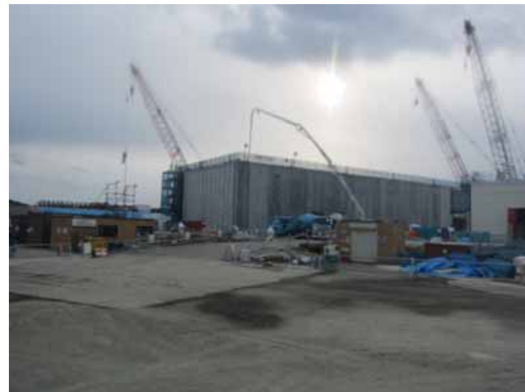
- 3 Waste sludge storage facility Jan. 9, 2012 photo by TEPCO staff
