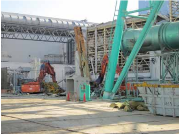
- 1 Removal of debris around Unit 3,4 Reactor Building Jan.10, 2012 photo by TEPCO staff
