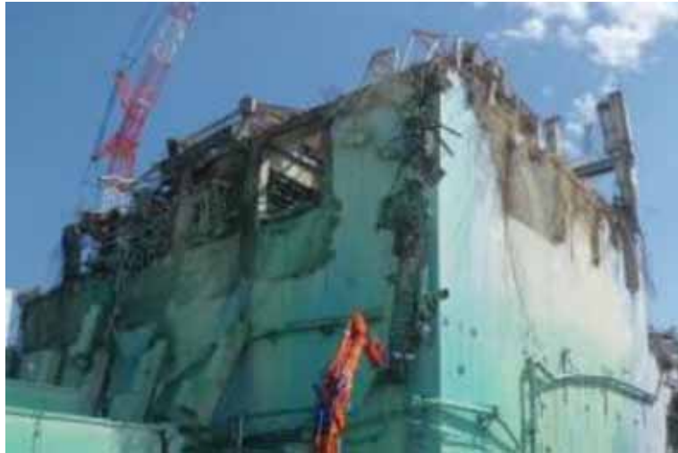
- 5 Removal of debris on the upper side of Unit 3 Reactor Building (before work)
