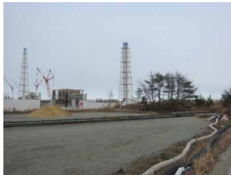
- 2 Look into Reactor Building from the hill in the southern side of Unit 4 Jan. 9, 2012 photo by TEPCO staff
