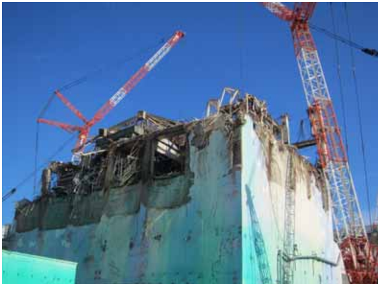
- 3 Unit 3 Reactor Building Jan.10, 2012 photo by TEPCO staff
