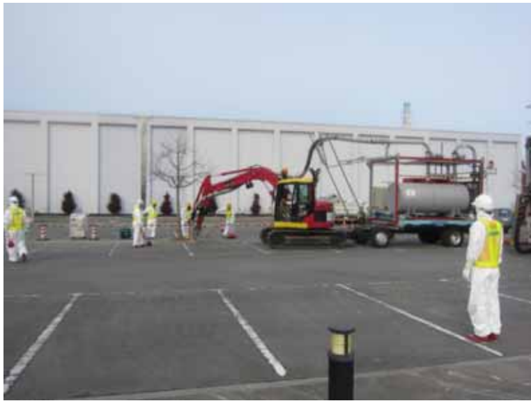
- 1 Collection work of dust and small debris at parking area of Main Anti-earthquake Building
