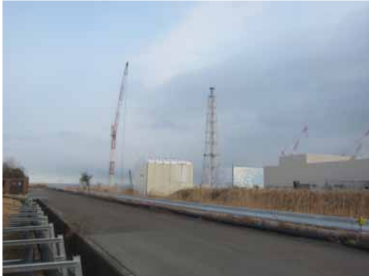
- 1 Look into Unit 1 Reactor Building from the backside of Main Anti-earthquake Building
