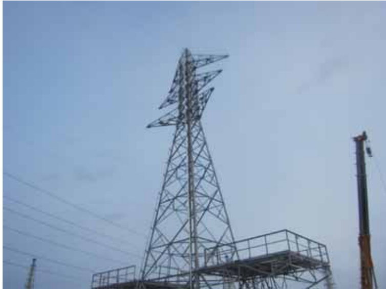
- 1 Lead-in tower from new switch station Jan. 9, 2012 photo by TEPCO staff
