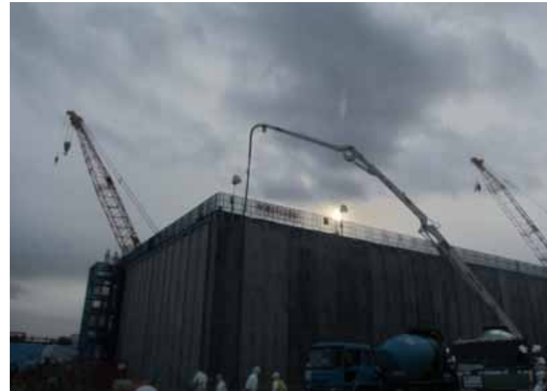
- 1 Waste sludge storage facility Jan. 9, 2012 photo by TEPCO staff
