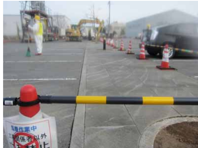
- 8 Collection work of dust and small debris at parking area of Main Anti-earthquake Building (after work)
