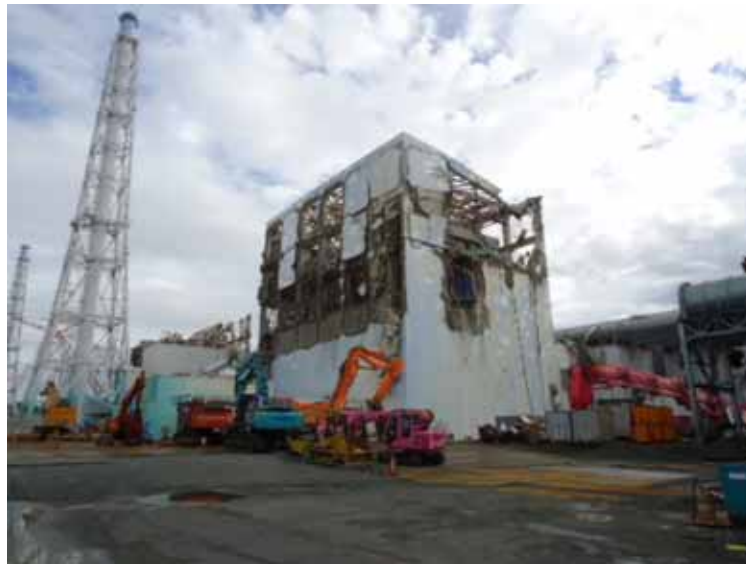
- 7 Removal of debris on the upper side of Unit 4 Reactor Building (before work)
