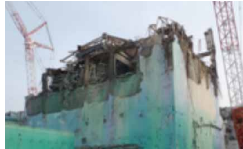
- 6 Removal of debris on the upper side of Unit 3 Reactor Building (after work)
