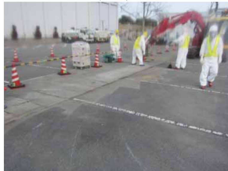
- 9 Collection work of dust and small debris at parking area of Main Anti-earthquake Building (after work)
