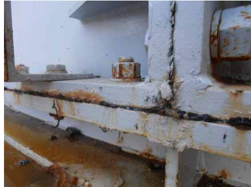
<Close-up photo of the leaked point>
