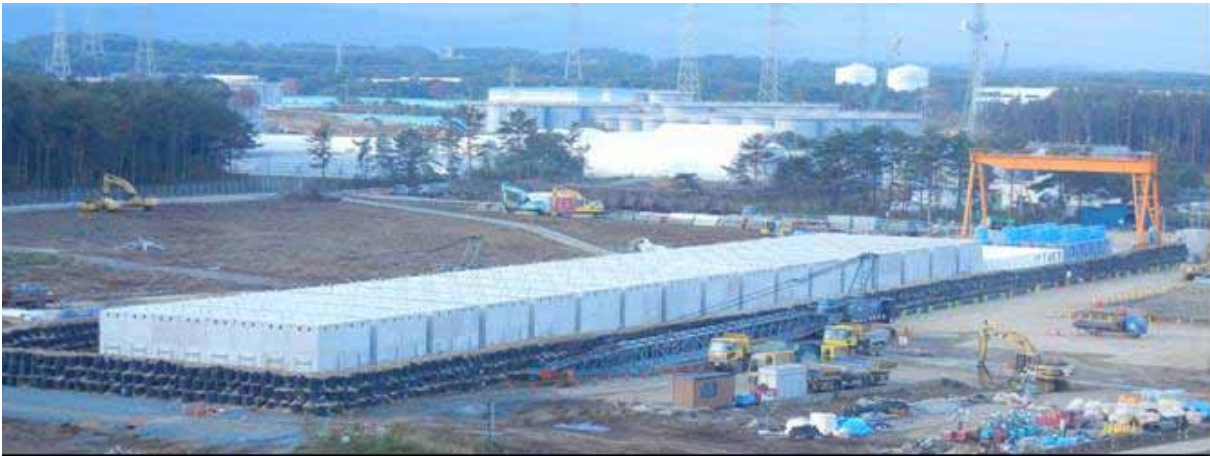
Overview of temporary storage for cesium adsorption towers
