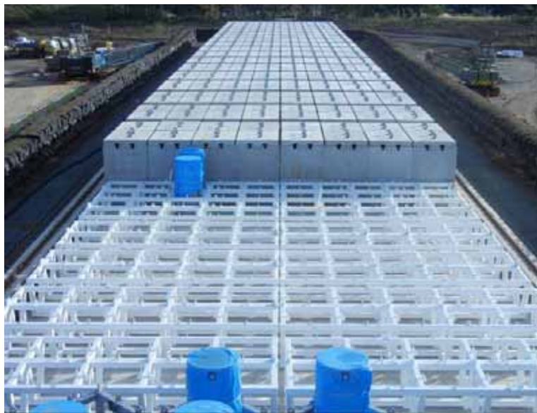
Temporary storage for cesium adsorption towers (Cesium adsorption towers covered by sheet are unused)
