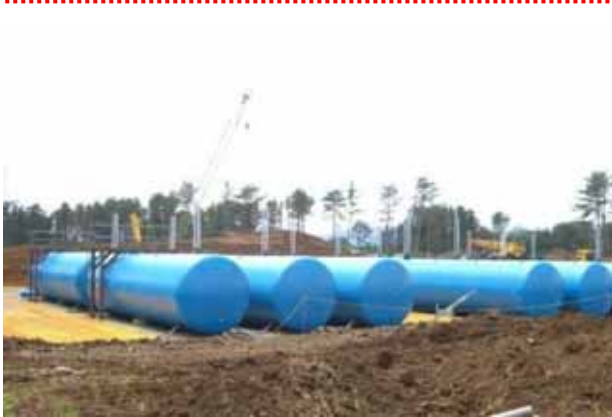
Tanks for highly concentrated accumulated water ( Placed underground due to the shielding )
