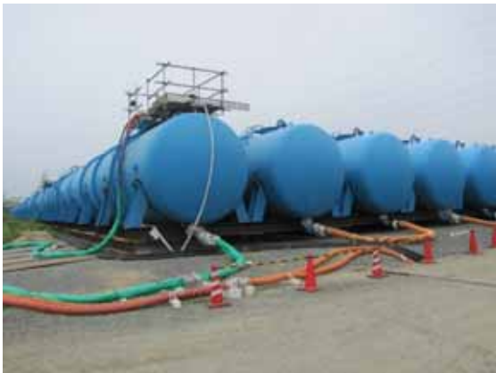
Tanks for concentrated waste water ( also Utilize for concentrated sea water )
