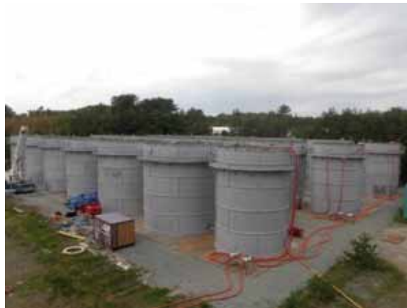
Tanks for low concentrated accumulated water
