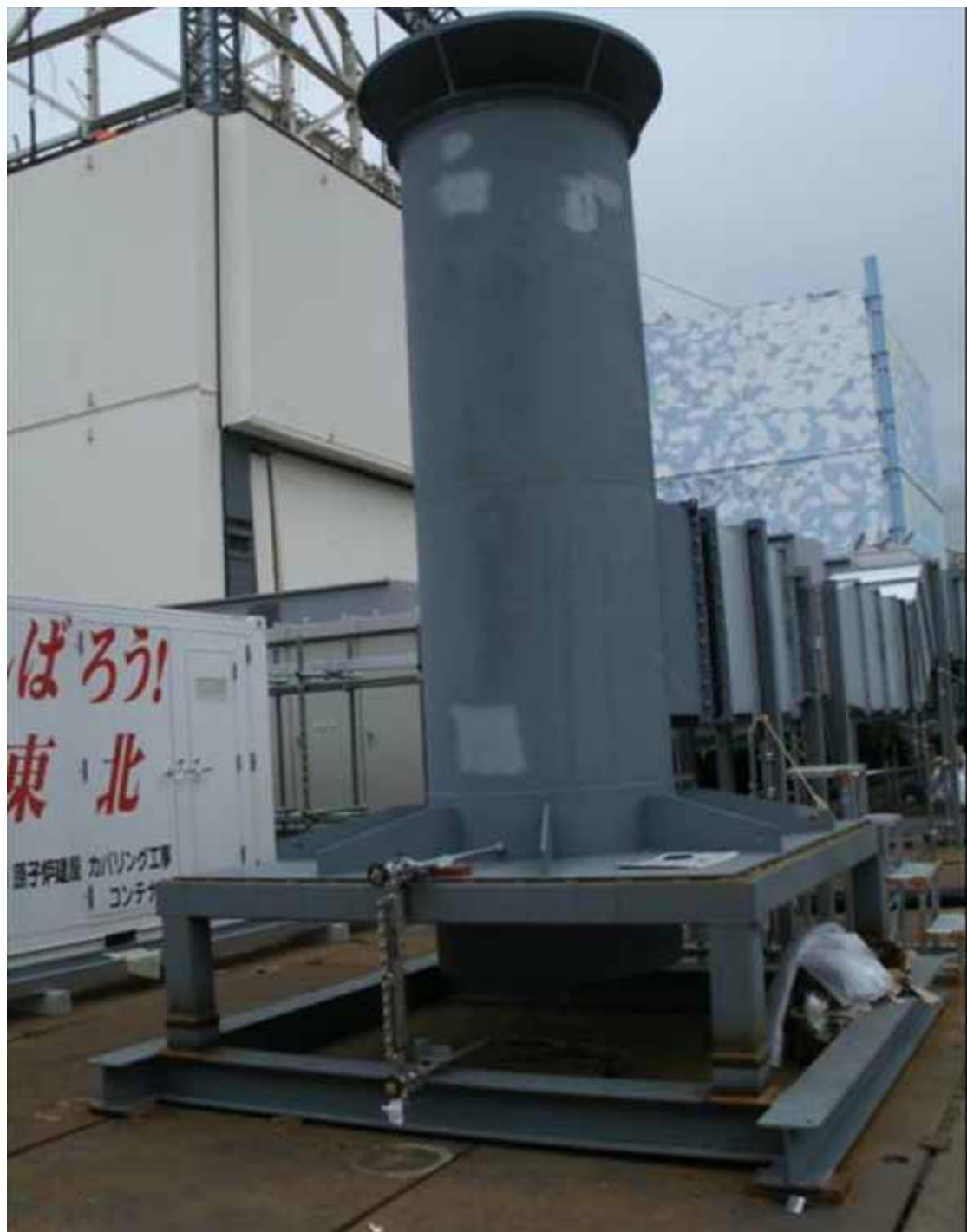
Exhaustion Tower [ September 27, 2011 Photo: TEPCO ]
