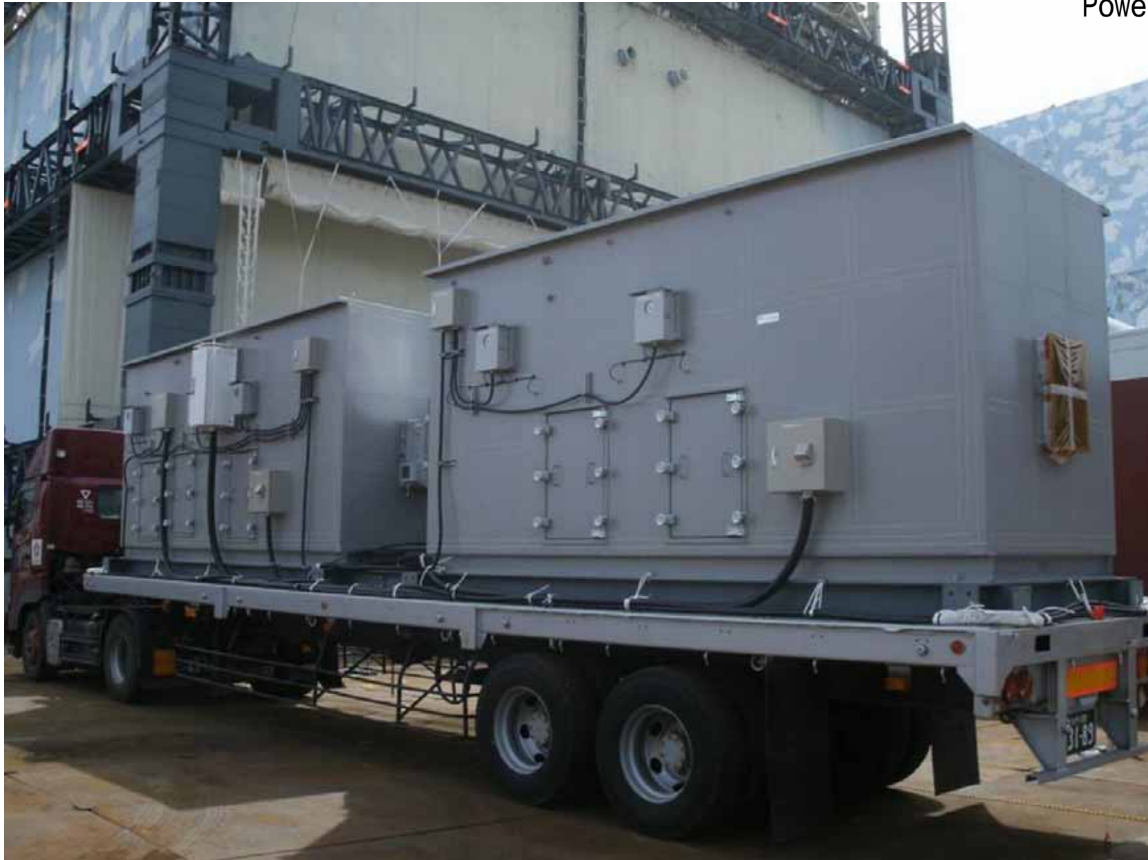
Filter Unit [ September 5, 2011 Photo: TEPCO ]
