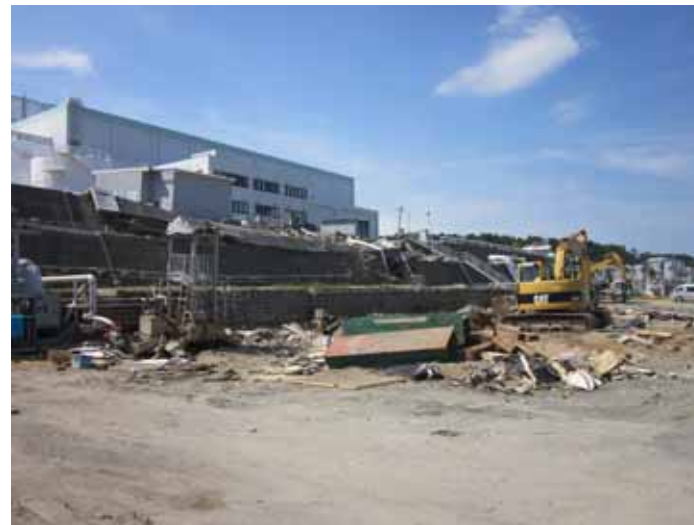
( 28 ) Unit 5 Seaside slope Taken by TEPCO employee on August 25,2011
