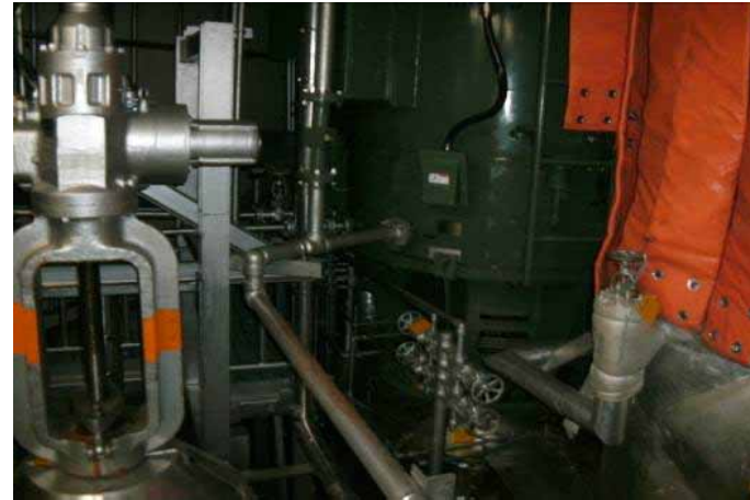
(2) Unit 5 residual heat removal system (RHR) pump (B)(D) (Reactor building B2F)
