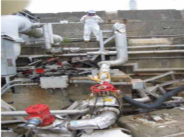
(37) Unit 5 and 6 Extinction pipes Taken by TEPCO employee on August 22,2011 (39)
