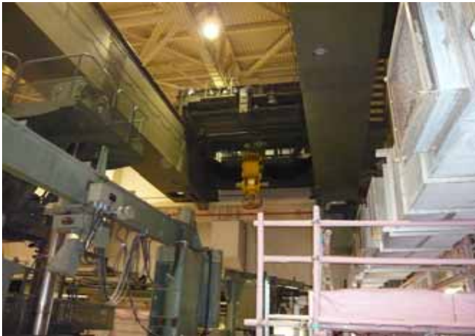
(3) Unit 5 Reactor building ceiling crane
