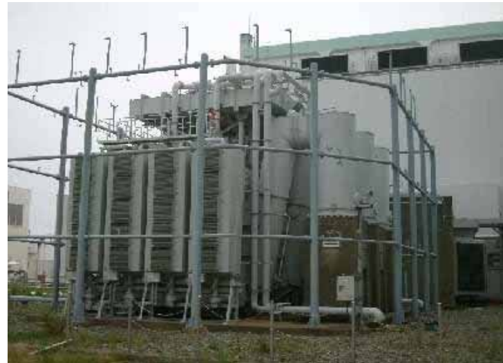
(36) Unit 6 Main transformer Taken by TEPCO employee on August 24,2011
