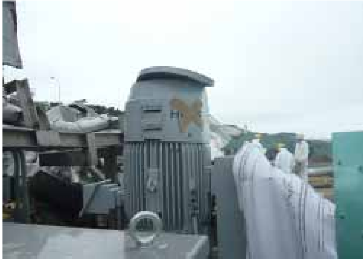
(33) Unit 6 High pressure core spray system Diesel generator Seawater system pump Taken by TEPCO employee on August 23,2011
