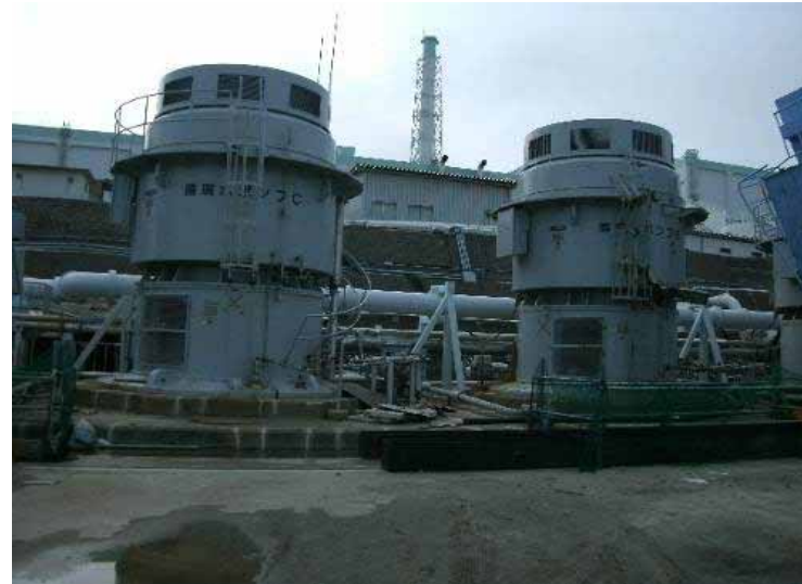
( 26 ) Unit 5 Circulating water pump (B)(C) Taken by TEPCO employee on August 23,2011
