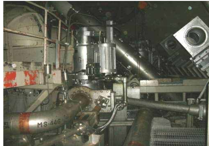
(4) Condition at Unit 5 Primary Containment Vessel 2F
