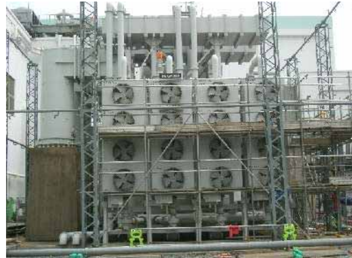
( 30 ) Unit 5 Main transformer Taken by TEPCO employee on August 24,2011
