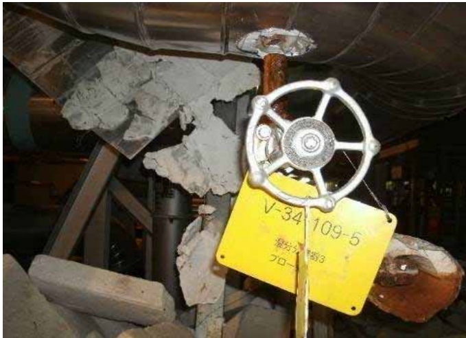
(7) Unit 5 Moisture separator(3) (Turbine building B1F ) Taken by TEPCO employee on August 23, 2011
