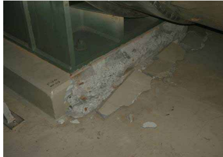
(22) Unit 6 feed water heater (Turbine building 1F) Taken by TEPCO employee on August 25, 2011
