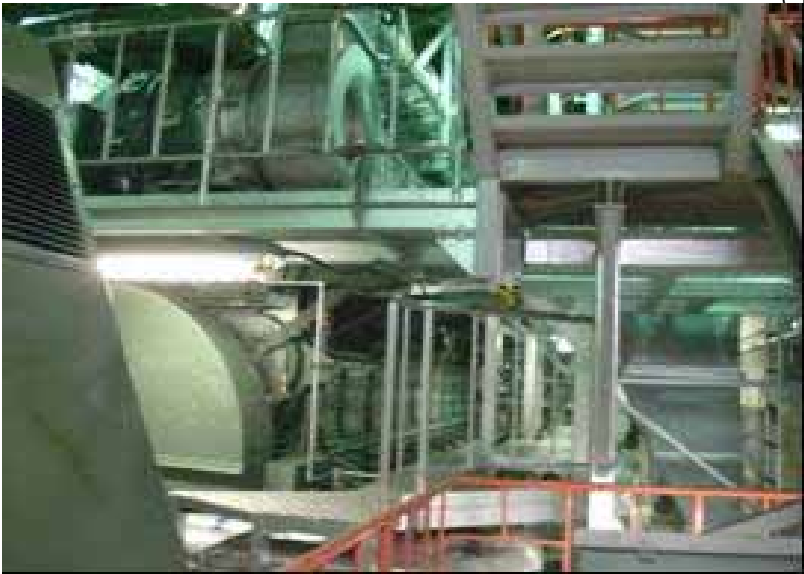
(14) Unit 6 Emergency diesel generator (A) (Turbine building B1F) Taken by TEPCO employee on August 19, 2011
