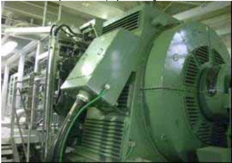
(15) Unit 6 High Pressure Core Spray System diesel generator (Reactor building B1F) Taken by TEPCO employee on August 19, 2011
