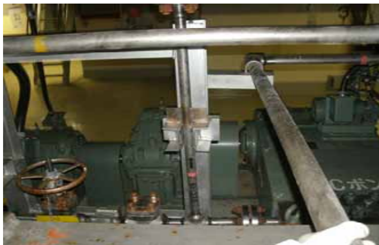
(19) Unit 6 Boric acid injection pump (A) (Reactor building 5F)
