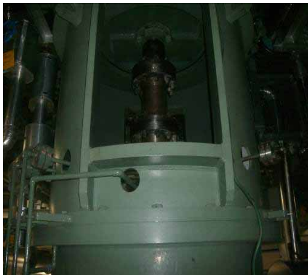
(17) Unit 6 Low Pressure Core Spray System pump (Reactor building B2F)
