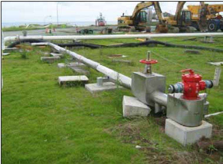
(38) Unit 5 and 6 Extinction pipes Taken by TEPCO employee on August 22,2011
