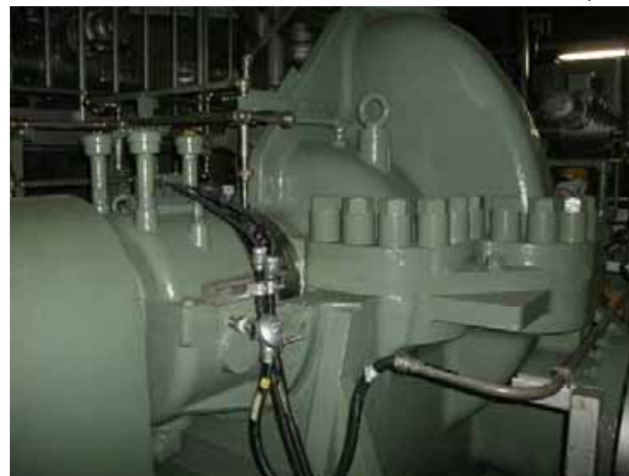
(20) Unit 6 High pressure condensate pump (Turbine building B1F)
