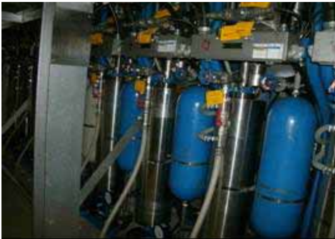
(11) Unit 5 Control rod water pressure control unit (Reactor building 1F) Taken by TEPCO employee on August 19, 2011
