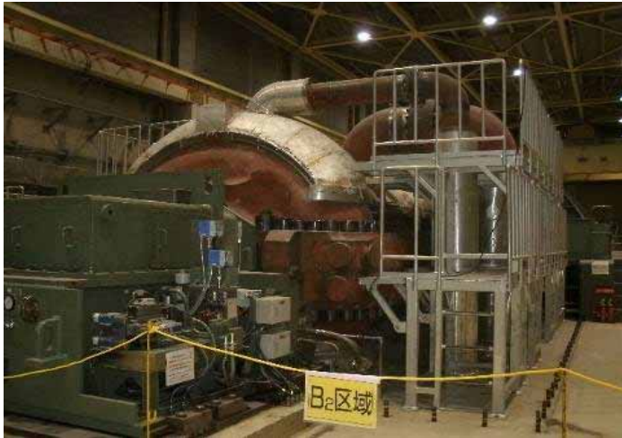
(9) Unit 5 High pressure turbine (Turbine building 2F) Taken by TEPCO employee on August 23, 2011
