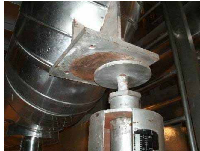
(8) Unit 5 Moisture separator drain pipe support (Turbine building B1F )
