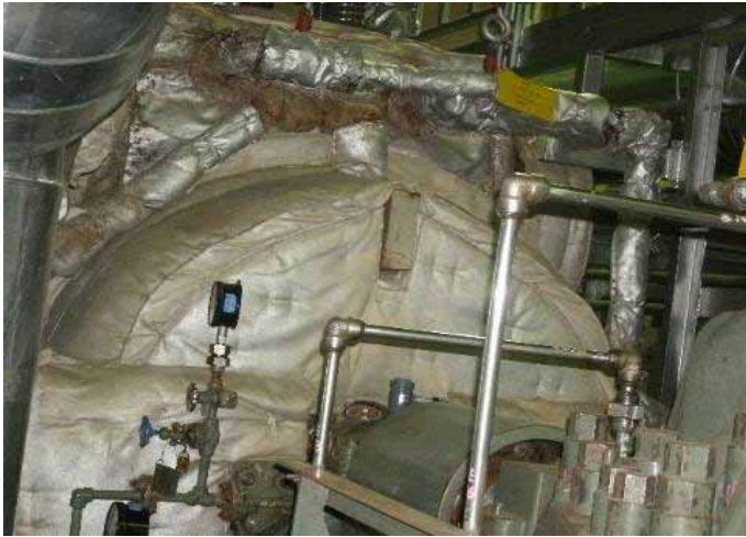
(1) Unit 5 High Pressure Coolant Injection System turbine (Reactor building B2F)
