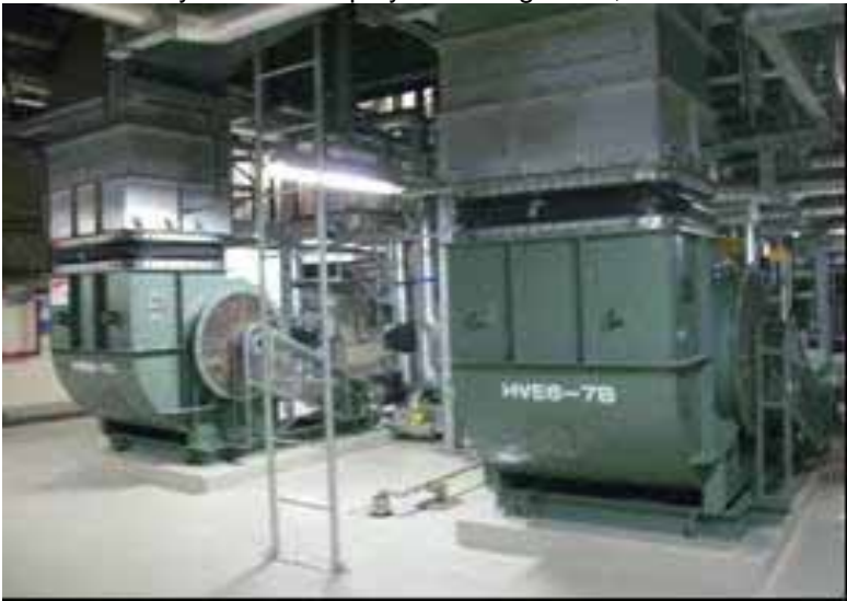
(16) Unit 6 gas treatment System (A)(B) (Reactor building 3F) Taken by TEPCO employee on August 19, 2011
