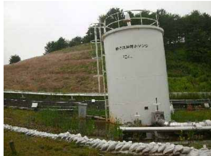
( 32 ) Unit 5 Insulator cleaning tank Taken by TEPCO employee on August 24,2011
