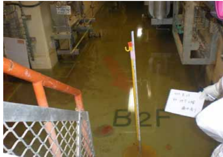
(24) Unit 6 Complex building B2F Taken by TEPCO employee on August 23, 2011
