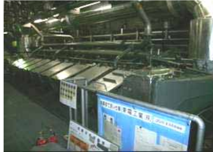
(6) Unit 5 Emergency diesel generator (Turbine building B1F)
