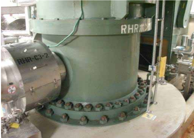
(13) Unit 6 residual heat removal system (RHR) pump (C) (Reactor building B2F) Taken by TEPCO employee on August 18, 2011
