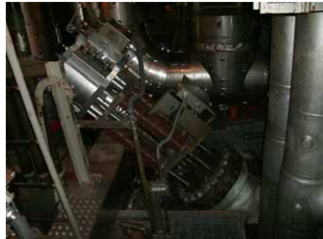
(12) Unit 5 Main steam isolation valve (Primary Containment Vessel 1F) Taken by TEPCO employee on August 17, 2011
