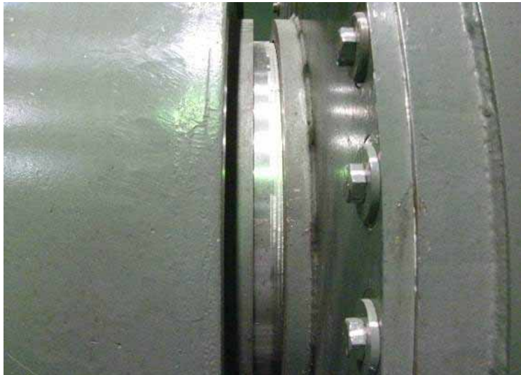
(23) Unit 6 Low pressure turbine (Turbine building 2F) Taken by TEPCO employee on August 23, 2011
