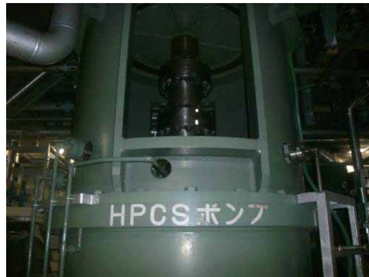
(18) Unit 6 High Pressure Core Spray System pump (Reactor building B2F)
