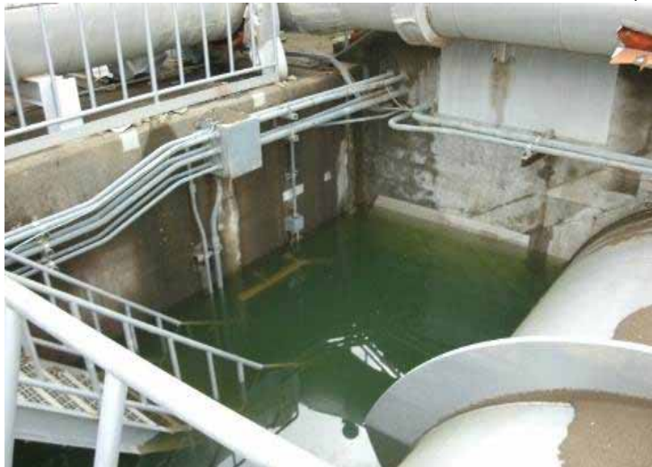
(35) Unit 6 Reversing valve pit Taken by TEPCO employee on August 22,2011
