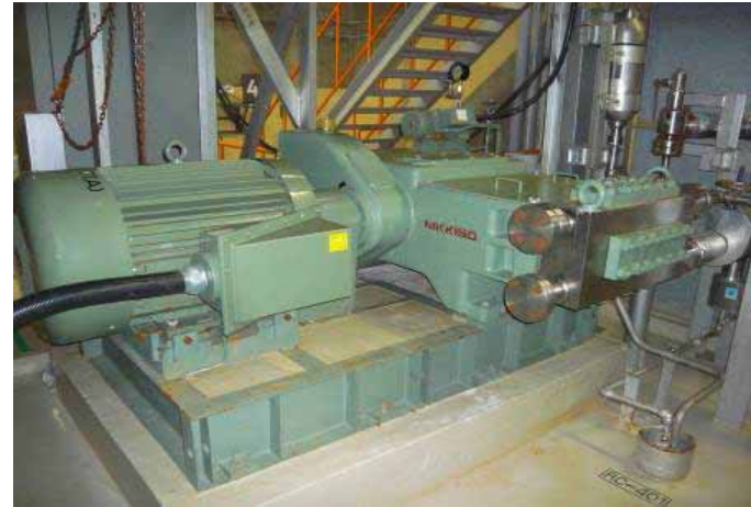
(10) Unit 5 Boric acid injection pump (A) (Reactor building 4F) Taken by TEPCO employee on August 19, 2011
