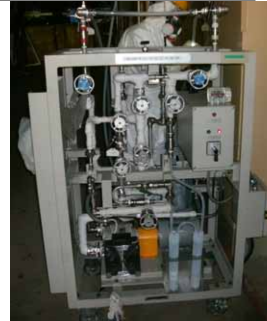
Fukushima Daiichi: Temporary gas sampling instrument for primary containment vessel (PCV) of Unit 1
