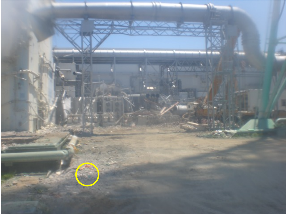
Small debris at Unit 3 west of R/B
