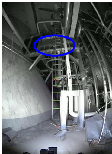
Grating at the valve of Core Spray System (point at ①)
