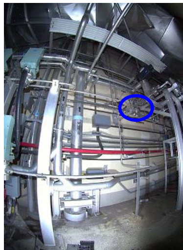
Valve of Water Supplement (Point at ②)
