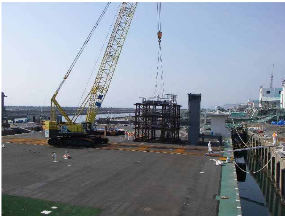
Photo: Tokyo Electric Power Company
