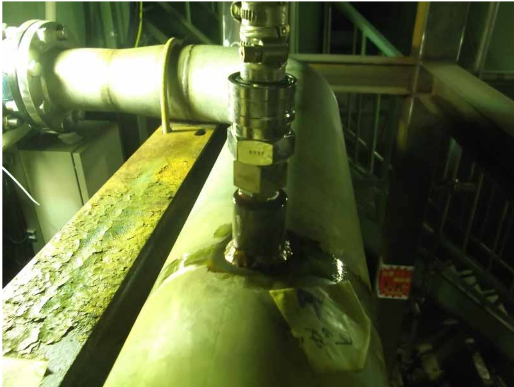
Hose Connection (before repair)
