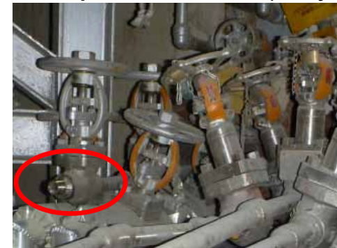
Nitrogen injection planned point ( after removing stoppage cap ) July 8, 2011, photo taken by TEPCO
