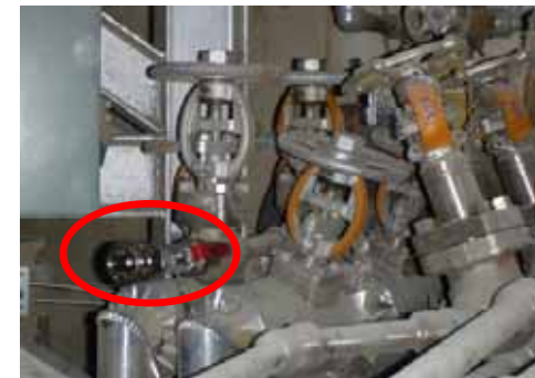
Nitrogen injection planned point ( after temporary fitting coupler ) July 8, 2011, photo taken by TEPCO
