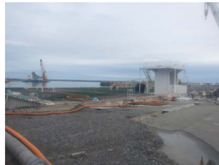
Megafloat tied up to around Shallow Draft Quay (Back of the picture)
