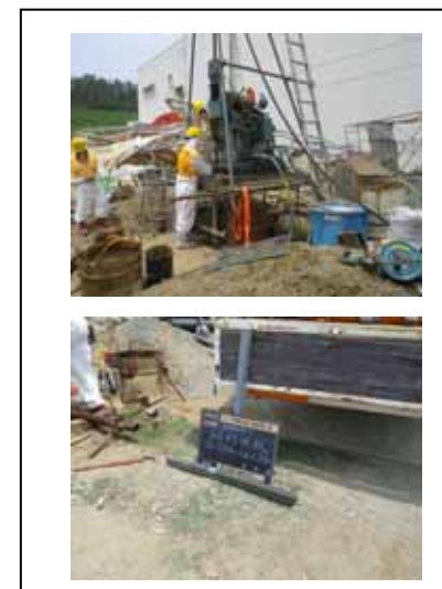
Pictures : Boring machine • collected samples Photo : Tokyo Electric Power Company Date : June 12, 2011
