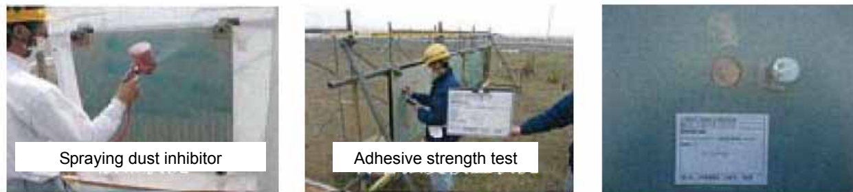
Figure 5: Spraying to the test materials and adhesive strength tests (steel plate surface)
