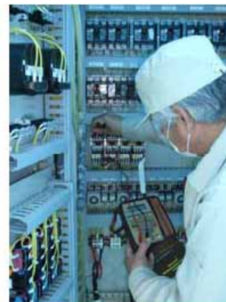
Insulation resistance test
