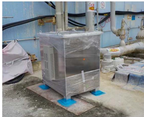
Unit 2 Muon transmission method (small-sized device) (Mar.-July., 2016)
