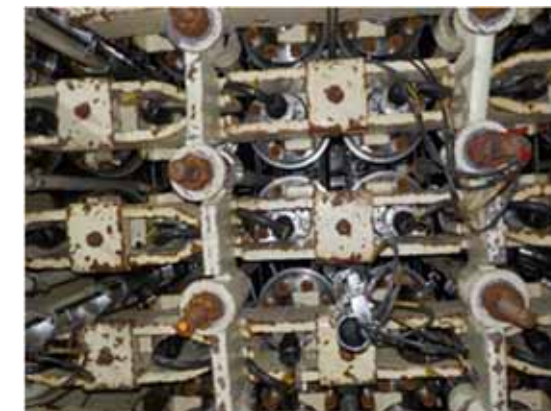
(ref) CRD housing at Unit 5 and CRD housing supporting clamp
