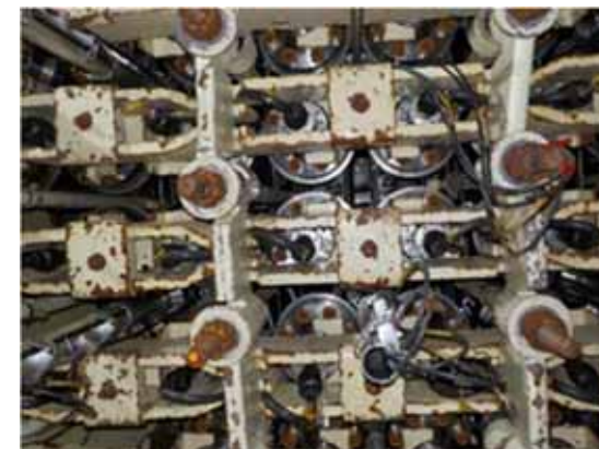
Reference: CRD housing and CRD housing supporting clamp inside the Unit 5
