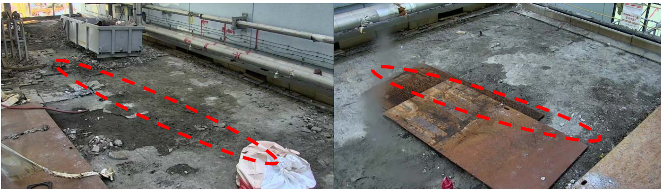
After Cleaning Up Rubble on the Small Attached Annex Installations of Pipes to Sprinkler Nozzles
