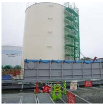
Temporary storage tank
