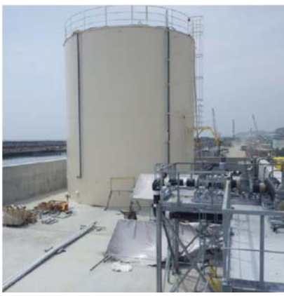
Water collecting tank
