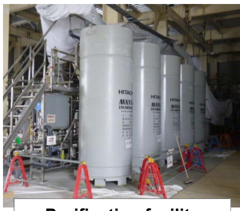
Purification facility (Adsorption tower)
