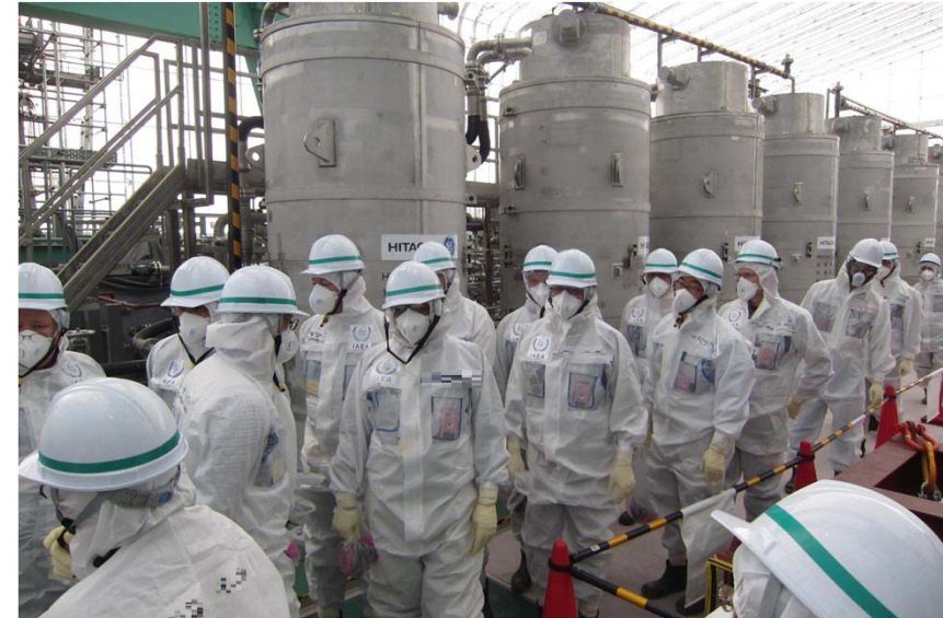
At the multi-nuclide removal equipment
