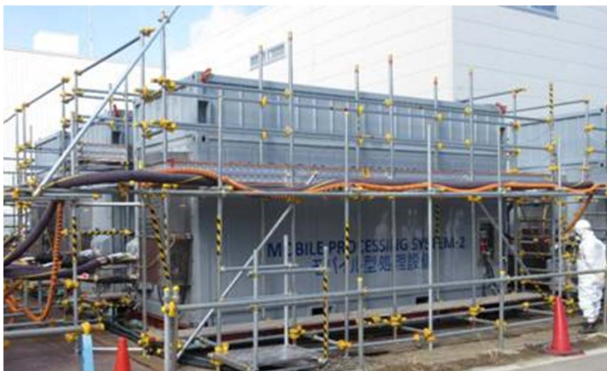
Mobile Strontium Removal Equipment (Unit B)
