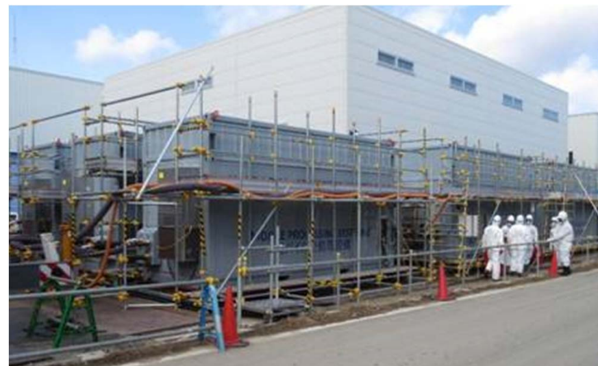
Mobile Strontium Removal Equipment (Unit B) Starting up activities for water treatment operation.
