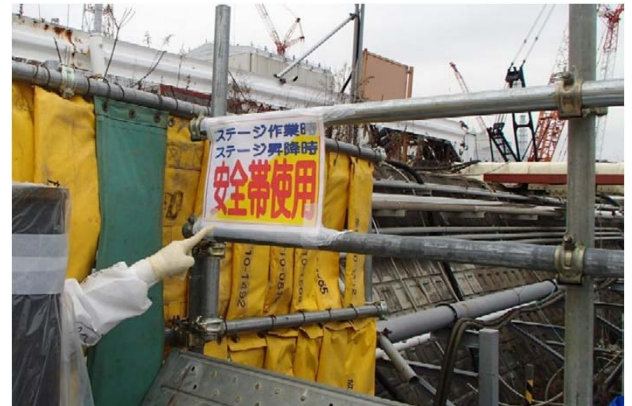
After the corrective action taken ("Use Safety Belt" sign was installed.)
