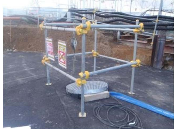
After the corrective action taken (barricade was set up around the opening. )
