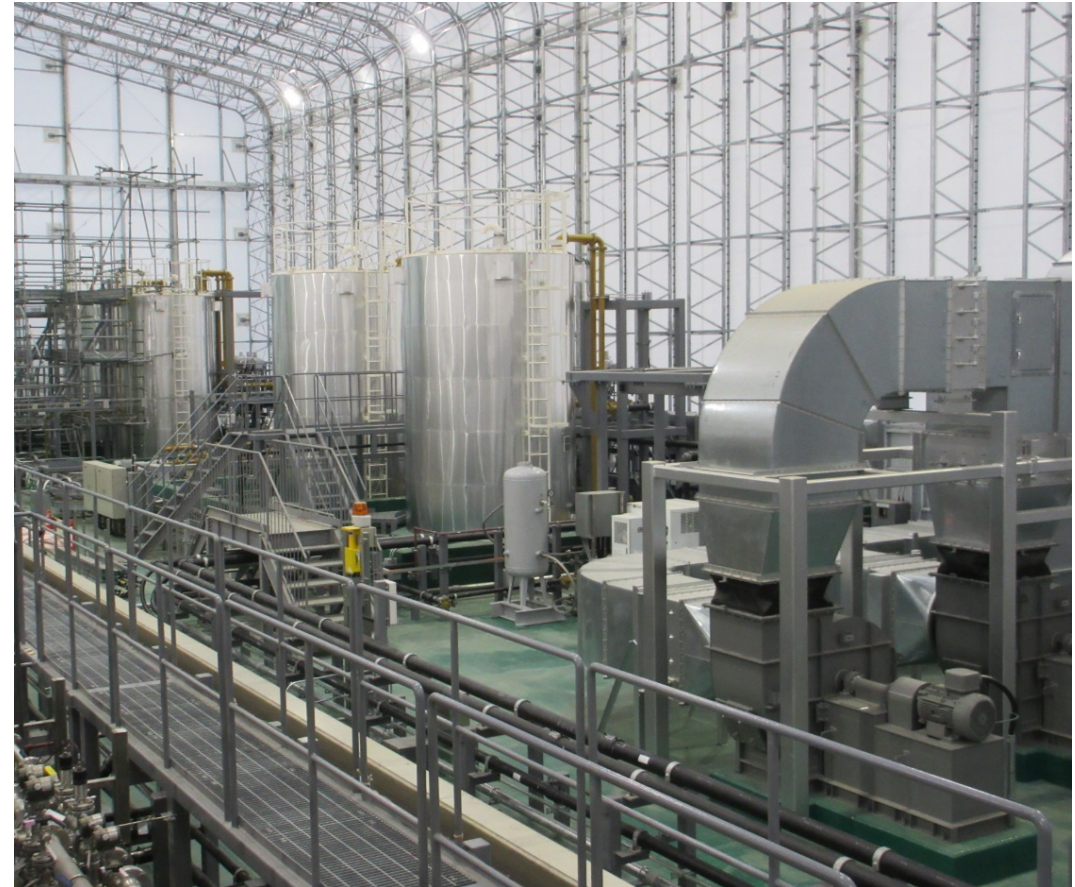
Treated water tank and Supply tank area
