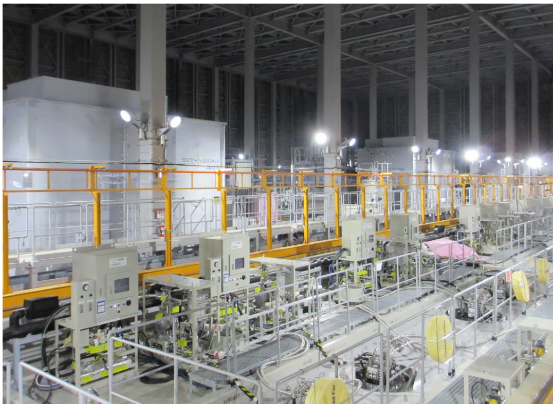
Cross-flow filter • HIC handling area
