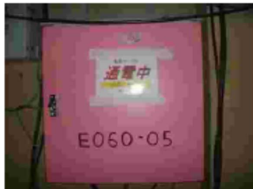
Temporary distribution board (1F, Incinerator workshop bldg.)
