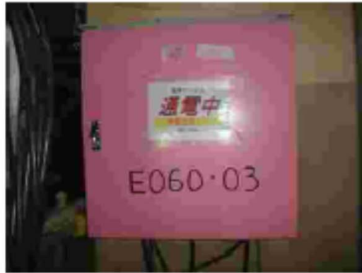
Temporary distribution board (2F, Process main bldg.)
