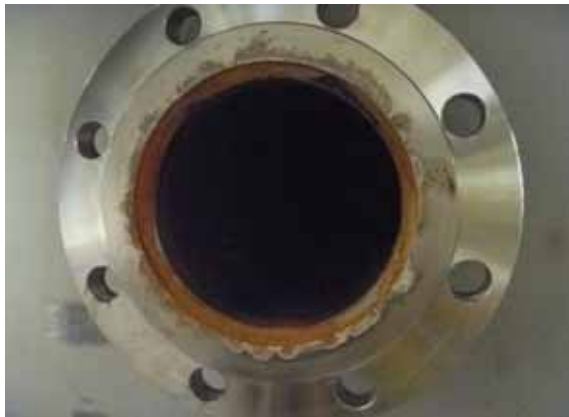
Batch treatment tank 2A decant nozzle with crevice corrosion on flange-sheet surface
