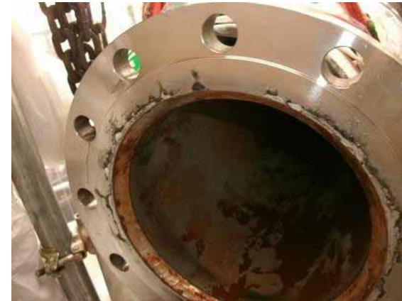
Circulation tank return pipe nozzle with crevice corrosion on flange-sheet surface
