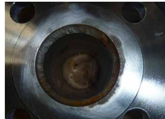
Supply pump 1A outlet pipe with crevice corrosion on flange-sheet surface
