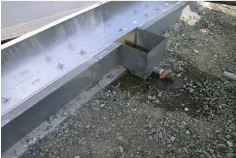
Leakage of water accumulated inside the H6 area dike
