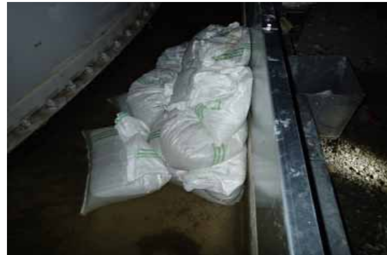
One temporary water stop measure to contain leakage of water accumulated inside the H6 area dike
