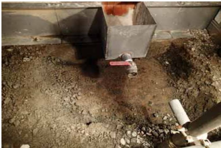
One temporary water stop measure to contain leakage of water accumulated inside the H6 area dike
