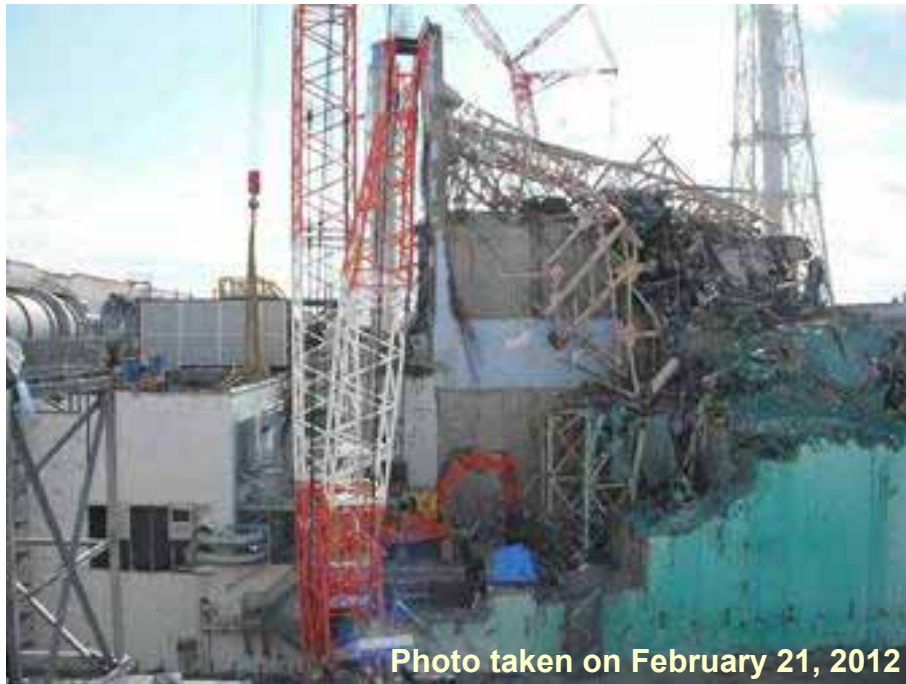
Before large debris removal
