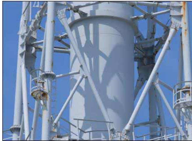
② East side (around 82-94 m above ground) Stack shaft of the exhaust stack
