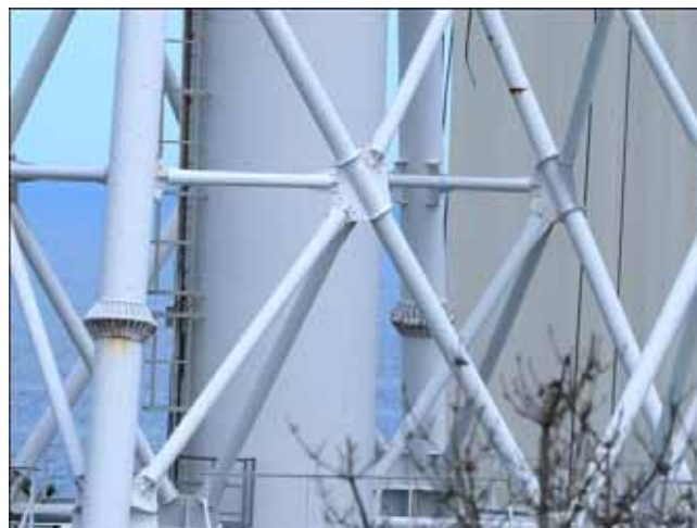
④ East side (around 19-30 m above ground) Stack shaft of the exhaust stack
