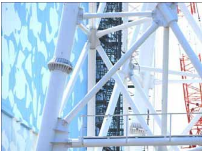
③ North side (around 19-30 m above ground) A principal post and diagonal bracings
