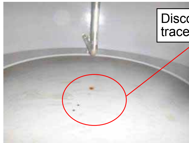
② Leaked-water receiving pan
