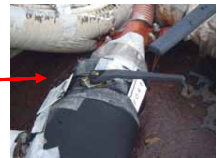
Main valve of treated water storage tanks (enlarged)
