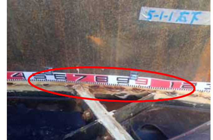
Packing slipping out on circumferential direction flange part (Photo taken on Sep. 19, 2013)
