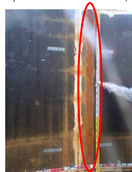
Rust generation on the side plate (1 st layer) (Photo taken on Sep. 19, 2013)
