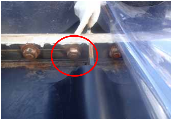
Loose bolt on the bottom-plate flange part (Photo taken on Sep. 19, 2013)
