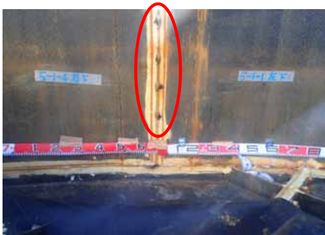
Packing slipping out on side-plate (1 st layer) longitudinal flange part (Photo taken on Sep. 19, 2013)
