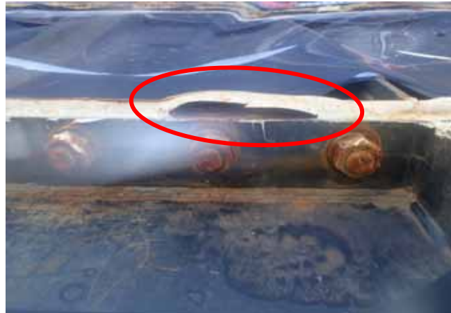
Swelling sealing member on the bottom-plate flange part (Photo taken on Sep. 19, 2013)
