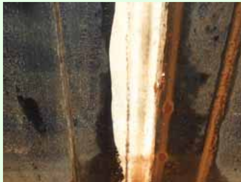
No.10 Gathering of rust at a side plate (Photo taken on Sep. 15, 2013)
