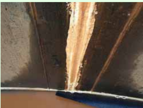
No.10 Joint between the side plate (1 st layer) and the bottom plate (inside) (Photo taken on Sep. 15, 2013)
