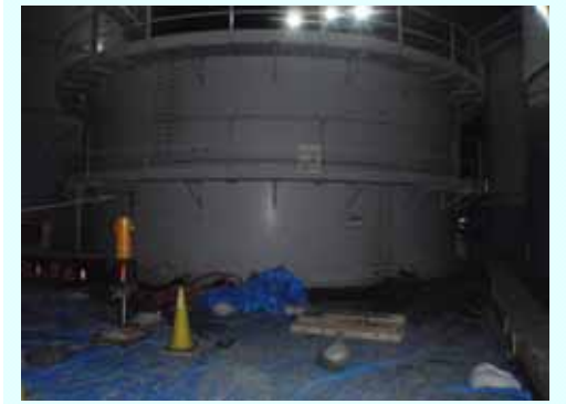
No.5 Completion of the side plate removal (3 rd layer) (Photo taken on Sep. 18, 2013)
