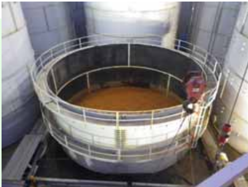
No.10 Completion of the side plate removal (3 rd layer) (Photo taken on Sep. 14, 2013)
