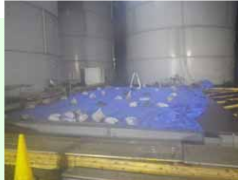
No.10 Completion of reinforcement for the bottom plate (Photo taken on Sep.16, 2013)
