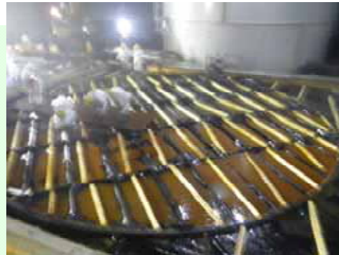
No.10 Completion of the side plate removal (1 st layer) (Photo taken on Sep. 16, 2013)
