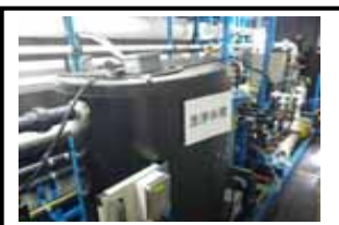
The point of overflowed (washing tank)
