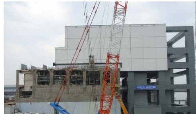
⑤ West wall (Outer surface)
