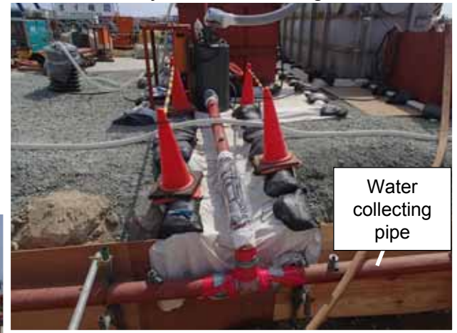
Connection of water collecting pipe Photo taken by TEPCO on August 15, 2013
