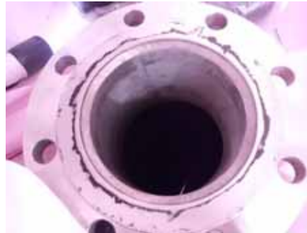
Flange surface (blank flange) of inspection port of the adsorption tower 1A
