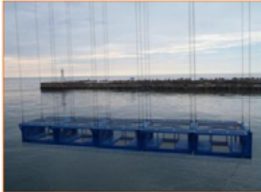
On July 11, installation of block fence at the port entrance was completed. (Photo: Installation work of the block fence)
