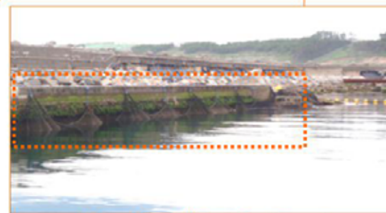
On June 26, installation of partition net around the south breakwater was completed.
