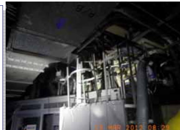
Conditions in upper space in R/B's 1st floor (Unit 2, as an example)
