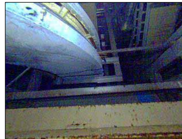
Photo taken at the upper side of the wall side of (4) (4.0m above the floor)
