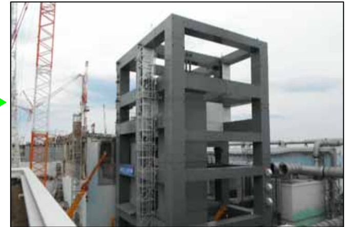
(3) Completion of the steel frame construction excluding the upper part of the Reactor Building (April 10, 2013)
