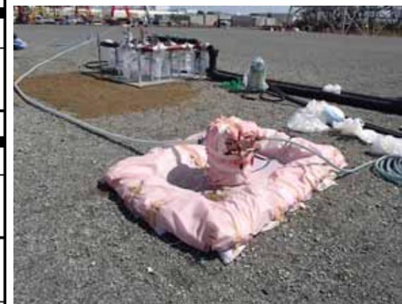
Installation of the pump at underground reservoir No. 3 (photo taken on April 13)
