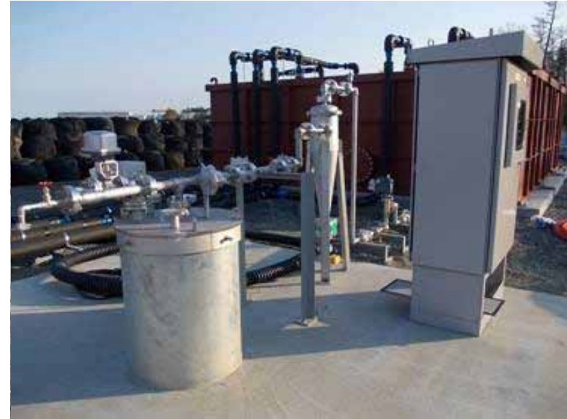
Pump well No.9 and the water pumping/transfer facility
