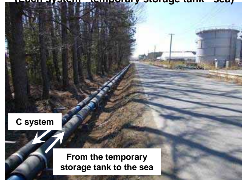
Transfer pipes (C system, temporary storage tank - sea)
