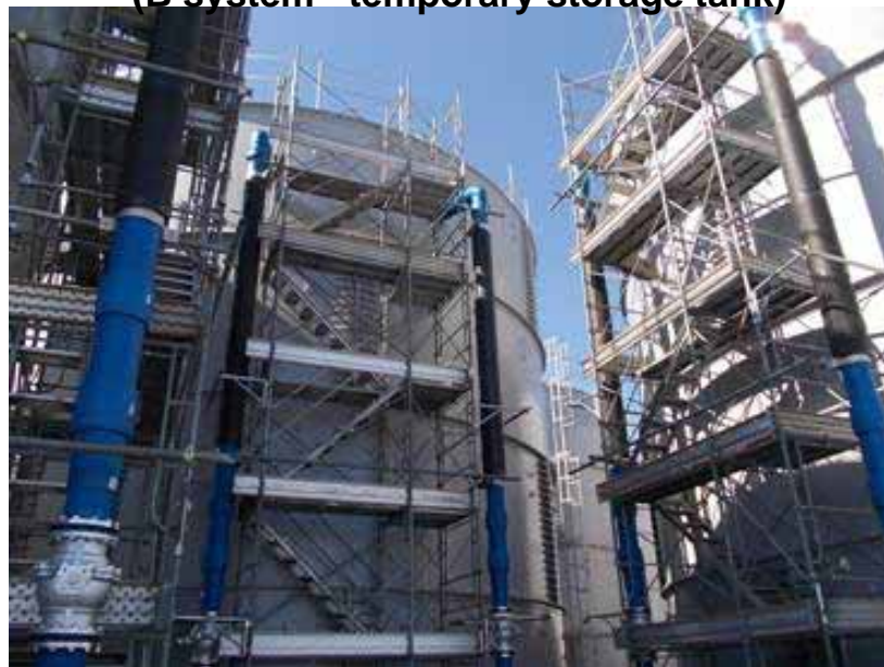
Temporary storage tank
