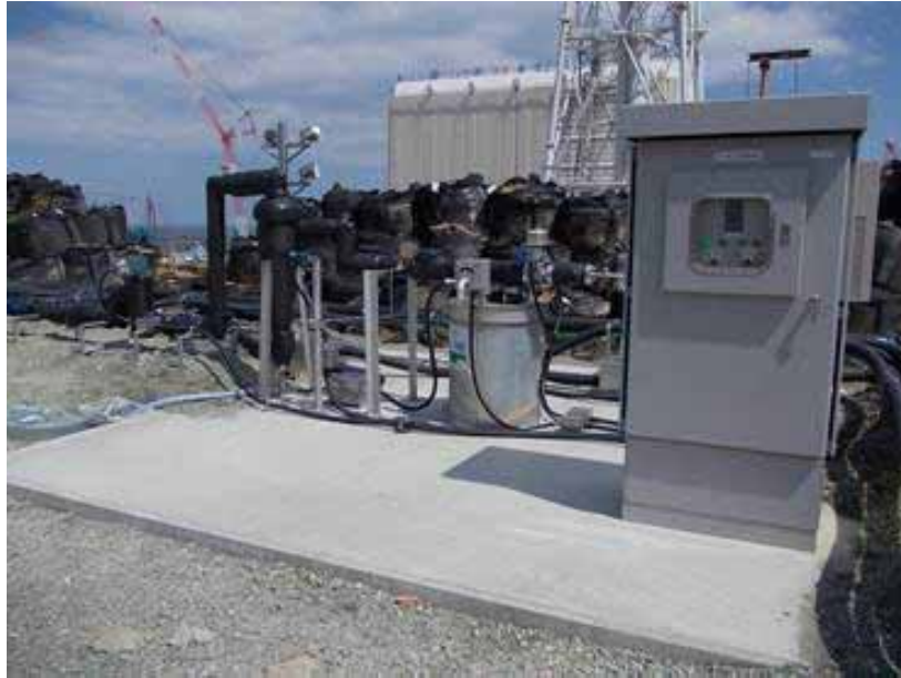
Pump well No.3 and the water pumping/transfer facility
