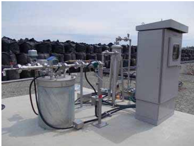
Pump well No.11 and the water pumping/transfer facility
