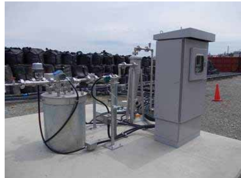
Pump well No.12 and the water pumping/transfer facility
