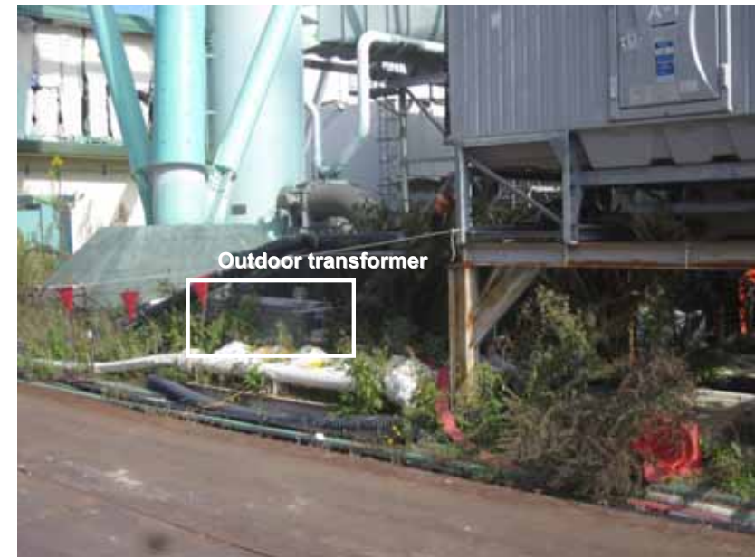
Photo 1: Outdoor transformer for Unit 2 spent fuel pool alternative cooling system at Fukushima Daiichi Nuclear Power Station
