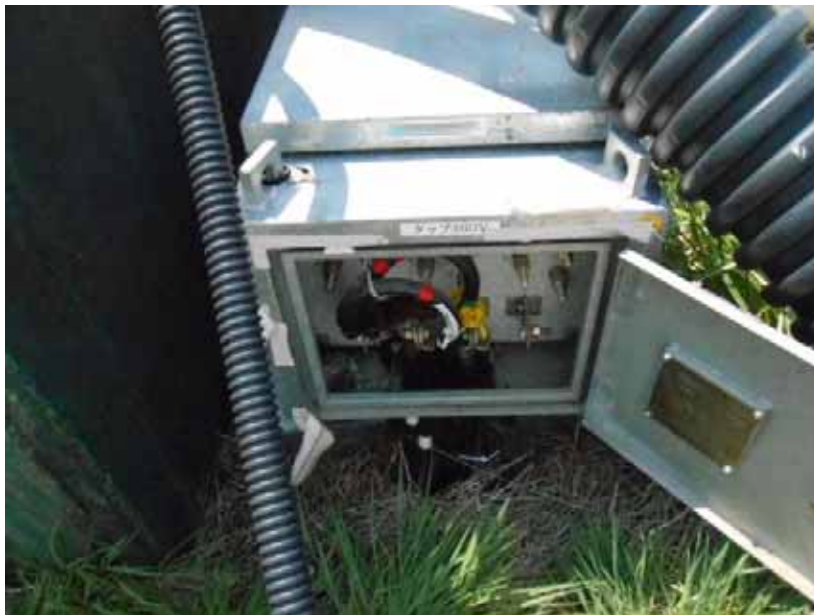
Photo 2: Outdoor transformer (Appearance)
