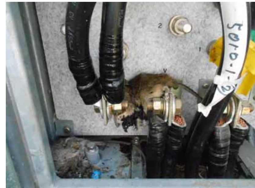
Photo 3: Outdoor transformer (Inside)
