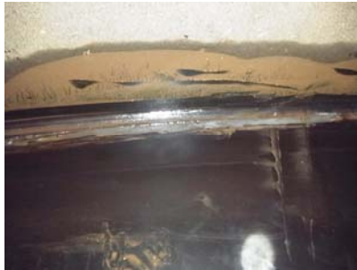
Paint coming off of the bottom plate
