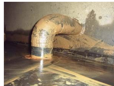
Trace of the drain pipe touching the bottom plate
