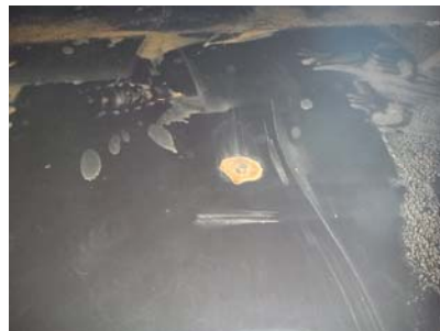
Paint bubbles in some locations of the bottom plate
