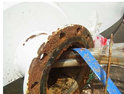
Corrosion of the spare nozzle flange
