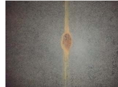
Paint bubbles in some locations of the side surface
