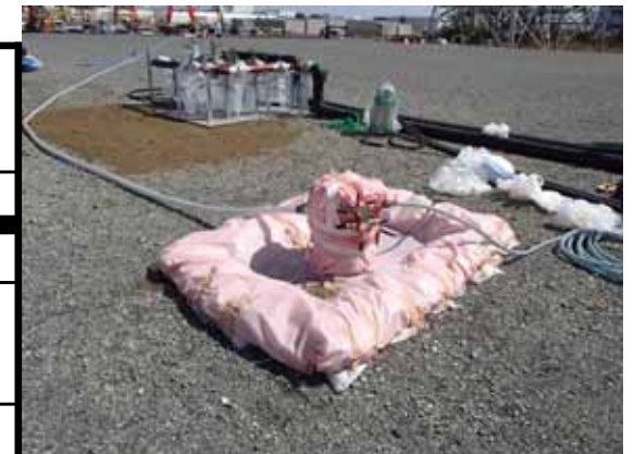
Installation of the pump at underground reservoir No. iii (photo taken on April 13)
