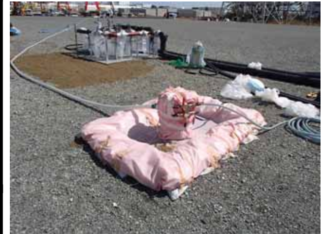
Installation of the pump at underground reservoir No. iii (photo taken on April 13)
